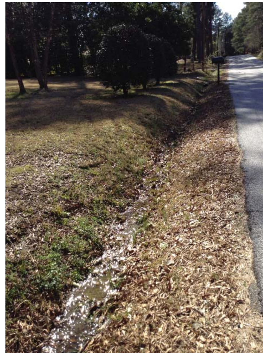
Queen Ann Street looking south, malfunctioning drain (50' ROW)
